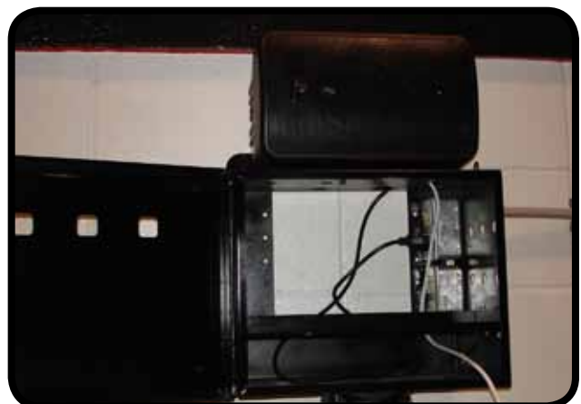
Properly installed speaker with power cord plugged into the outlet and audio cable routed under the shelf.
